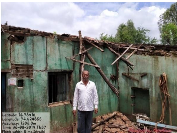
Visit at Flood Affected Area (Shirol)
